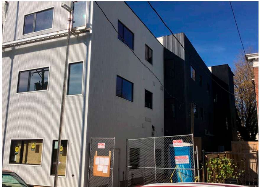
Constructing this building on a small side street in Philadelphia created many logistics challenges for Equinox Management and Construction.
