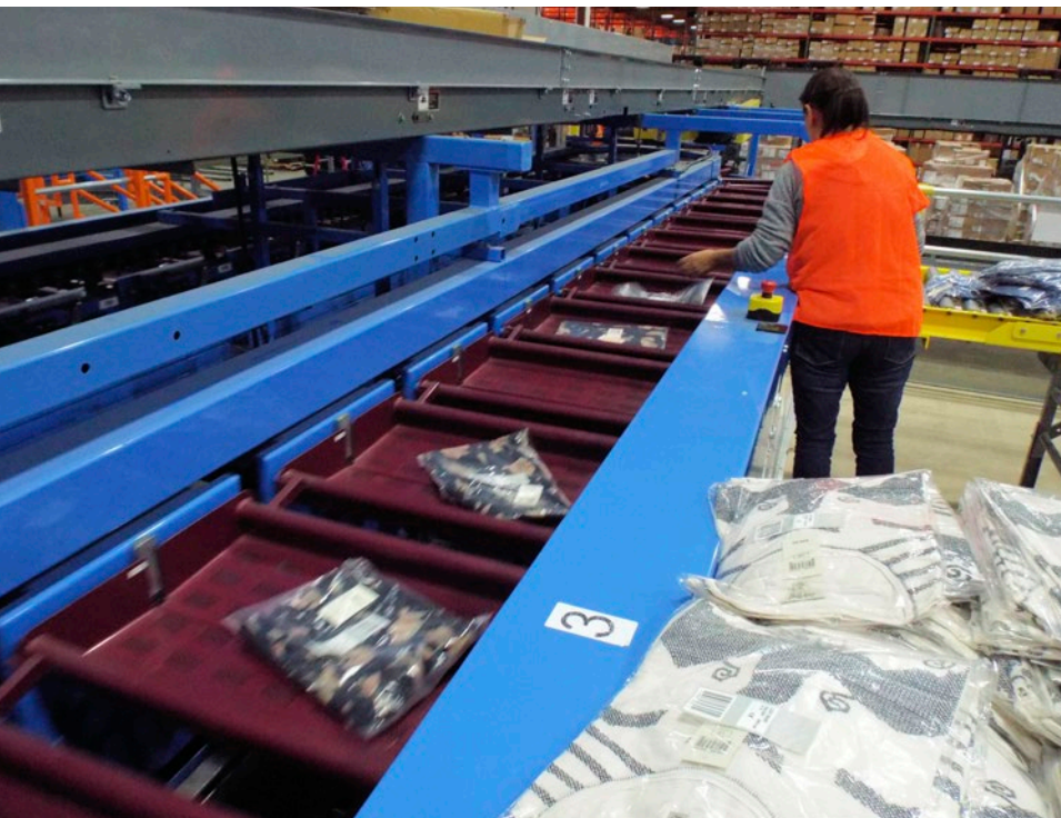
An existing Taylored Services distribution center was outfitted with new automation and materials handling solutions to provide Lucky Brand with fast order fulfillment.
