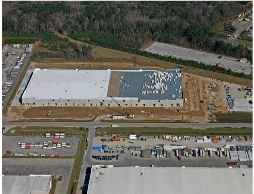
Construction is underway on a new 315,000-square-foot building in the CenterPoint Intermodal Center-Savannah, located just four miles from the Georgia Ports Authority. The facility provides shippers with the ultimate location advantage for goods distribution.
