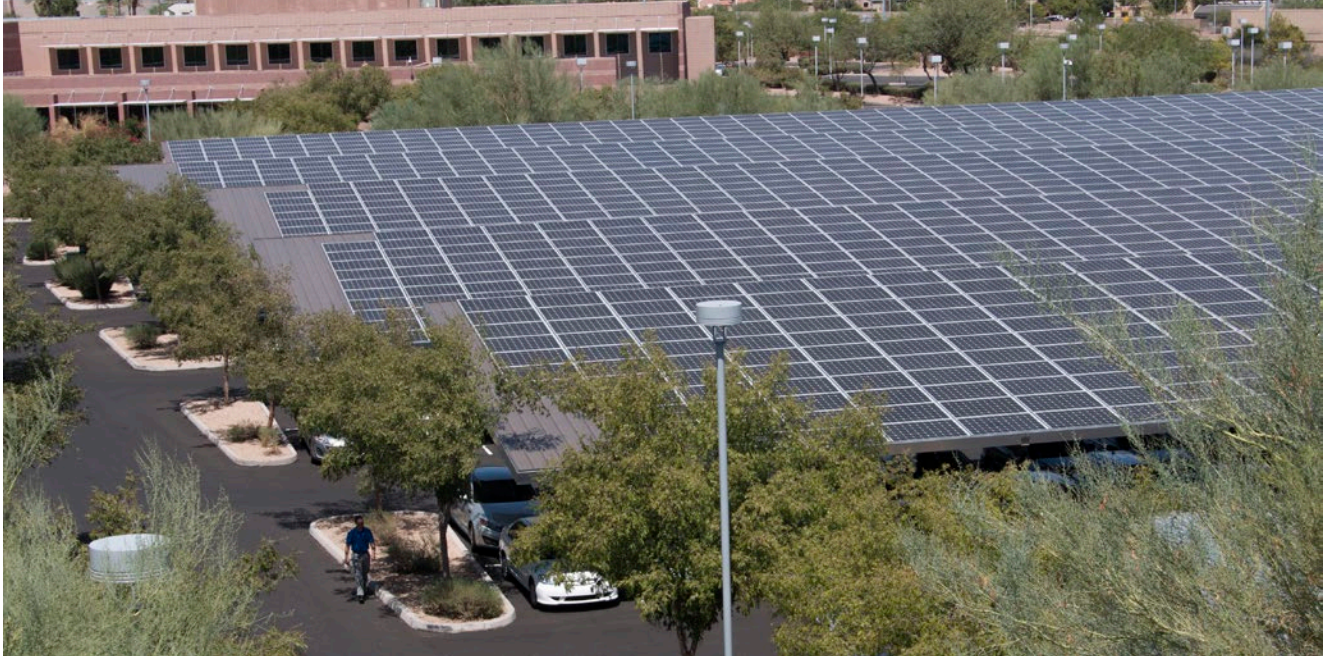
Avnet flipped the switch on a 1,000-kilowatt, 3,724-panel solar project that provides approximately 60 to 65 percent of the energy for its headquarters in Tempe, Ariz.
